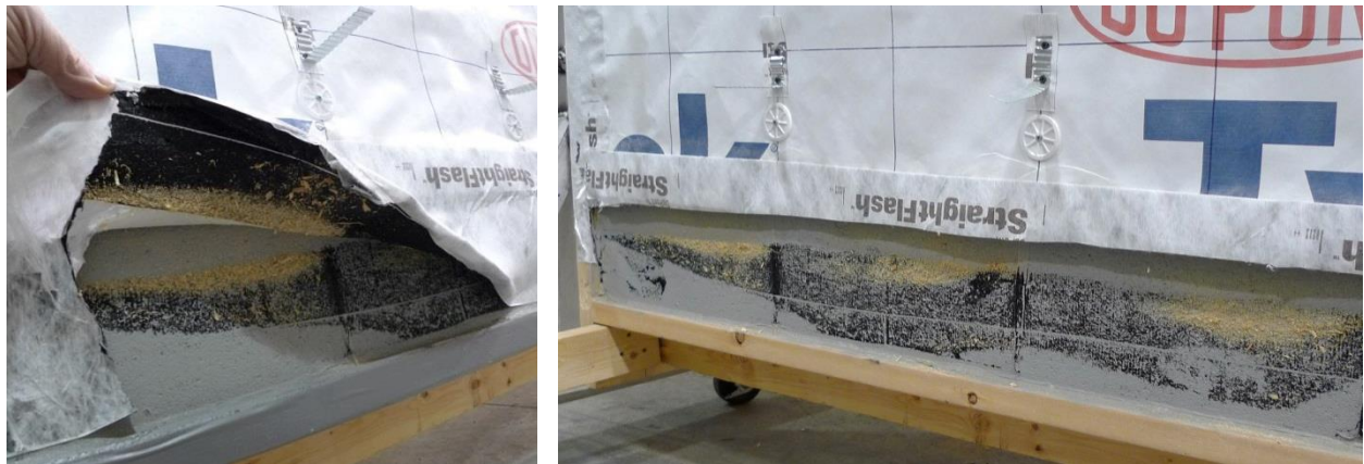
Figure 19. Failure of the flashing tape adhesive.
