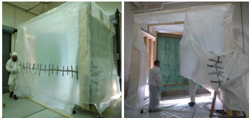
Figure 31. Enclosed and ventilated area built to contain emissions during spray foam installation.
